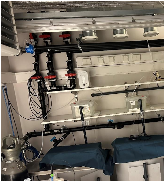
Figure 3: injection of Carbon dioxide from the flask into water by diffusor.
