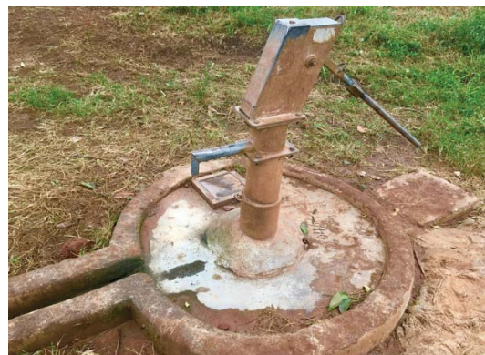
Figure 2.3 The manual hand pump with the shallow well
