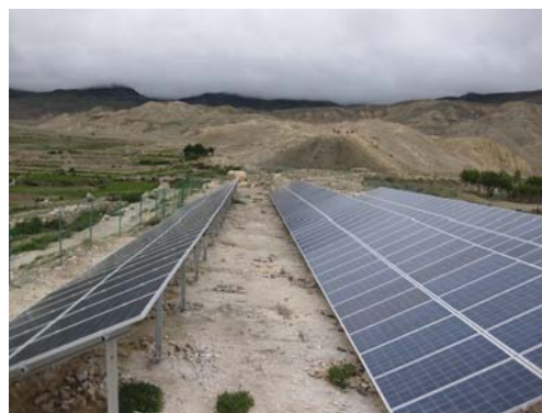
Figure 26: Solar power plant in Lo Manthang
